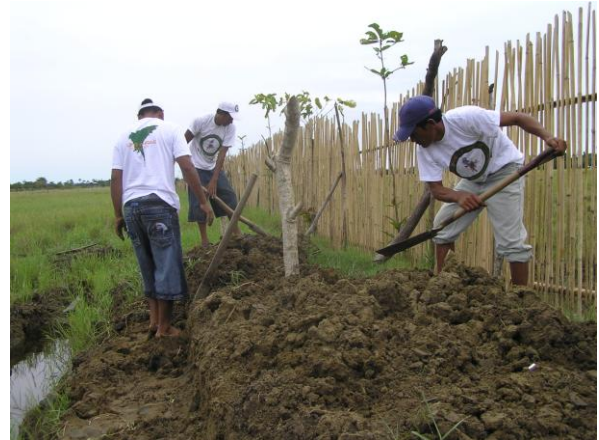
Figure 3: Temporary bamboo fence and adjacent drainage channel along the boundary line of the entire 2 ha area. ©SSchoppe
