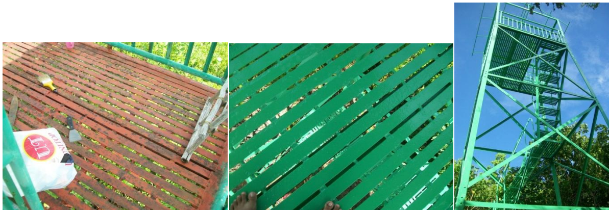
Figure 9. The left side picture shows the platform before it was repainted and the middle photo shows the same platform after removing rust and repainting was completed. The tower is ready for visiting guests and birders. ©KFI
